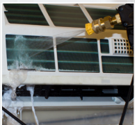
Clean coils from the front
